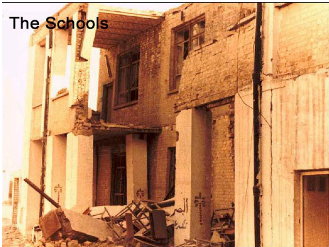
Figure 2 : School damaged during the US-UK aggression on Iraq in 1991[13]
