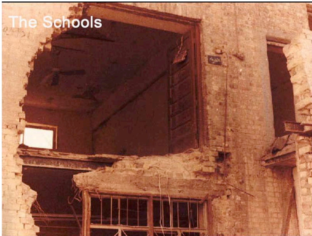
Figure 1 : School damaged during the US-UK aggression on Iraq in 1991 [13]
